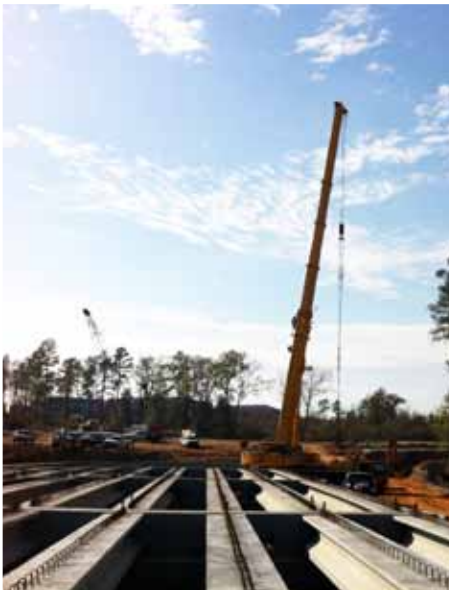
The bridge is a six span structure that measures 408 feet long X 76 feet wide and included 60 – TX34 concrete beams
